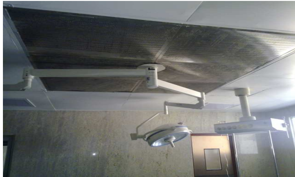
Picture - 1. Air -Filters – Operation theatres
